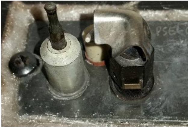
Figure 29 – Pilot in LP (slide gate to rear of Pilot Tower)
